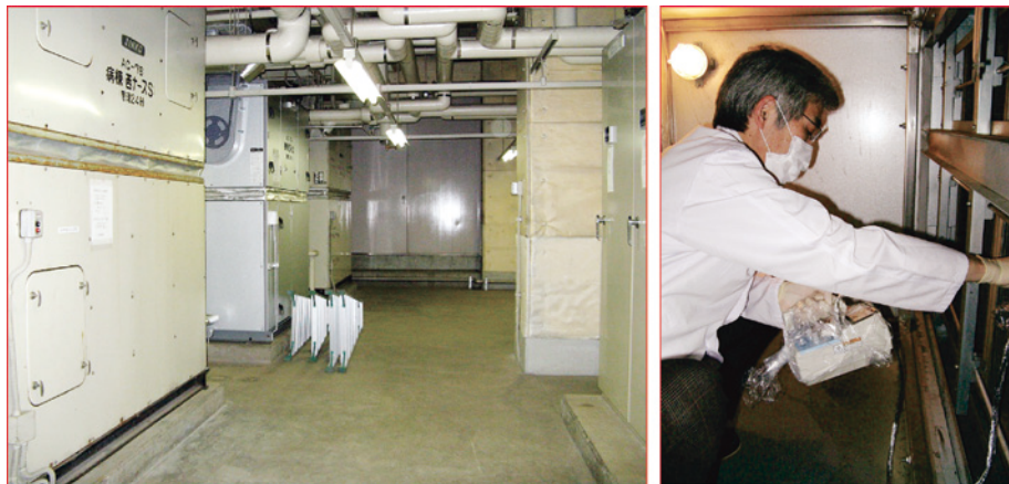
Fig. 3 Radiation survey at air conditioning room and air filter Radiation survey showed that many of the radioactive substances had been captured in the air conditioner filters.
